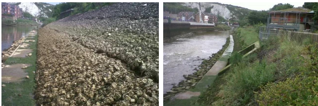
Plate 2-3 – Rock roll mattresses at Railway Lane, Lewes showing development of intertidal habitat over time (images courtesy of Salix)
