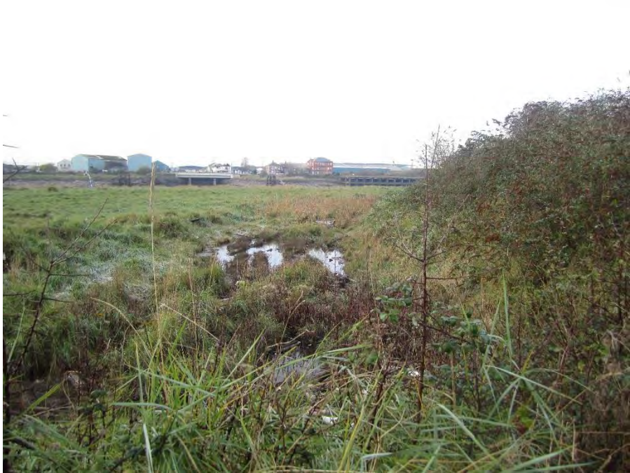
Figure 4 – Rutting and standing water at toe of embankment. View looking northwest along the embankment towards Point A.
